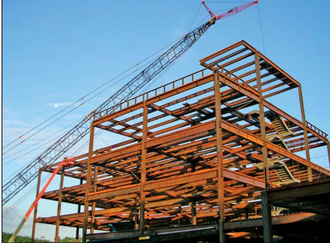
Facing a very tight construction schedule, Mercy Health Partners incorporated a Structural Engineer and Fabricator/Erector into the planning team. Design began in January 2005 with the initial architectural concept drawings. Erection of the main steel framing was completed in October 2005 - ten months from architectural concept to final bolt-up. Mission accomplished.
