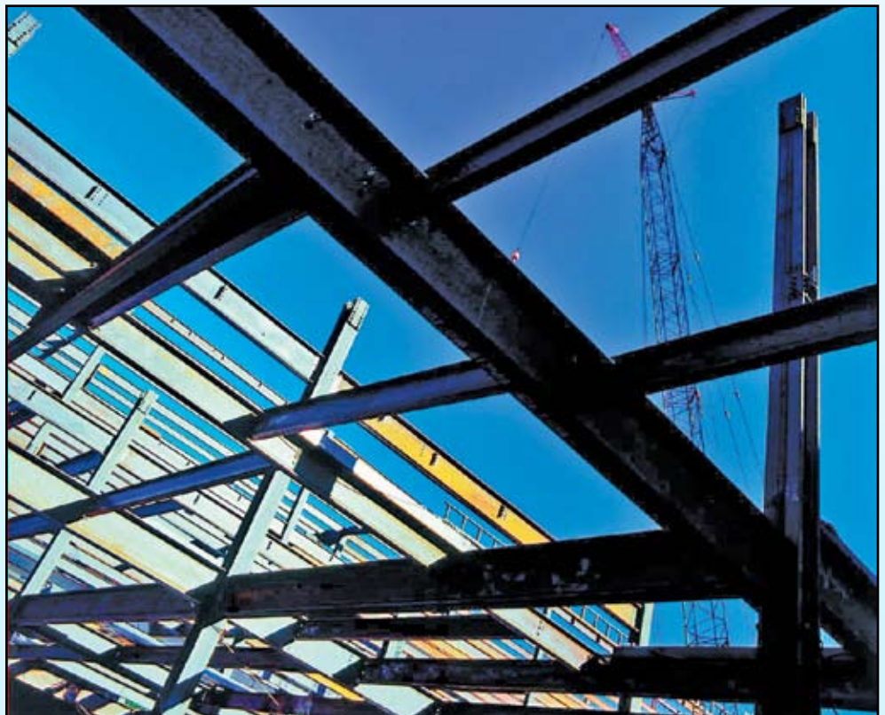
Using Constructability principles, the Mercy Heart Center Design/Build team shaved 16 weeks from the schedule and 140 tons of steel from the structure of the four-story, 144,000 square foot facility.
